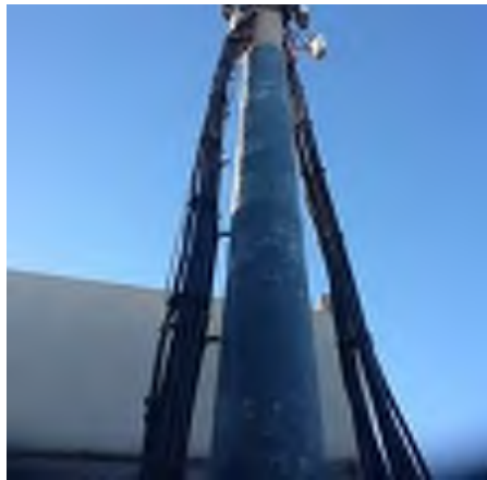
Carbon and glass FRP applied to the lower portions of the pole.
